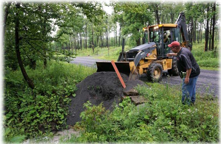
Figure 184 – Tom Clark directs DCNR as limestone sand is placed in Babcock Creek
